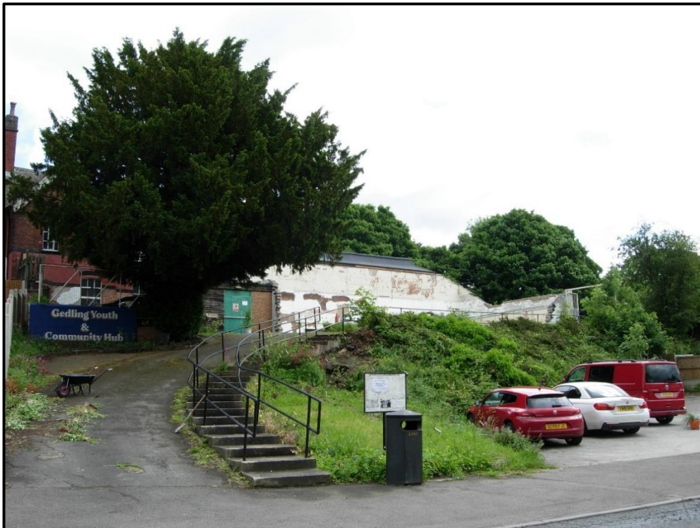
Photos: Gedling Station and car park following demolition of the modern extension partly implementing the planning permission and the rear of the Station and platform below.
