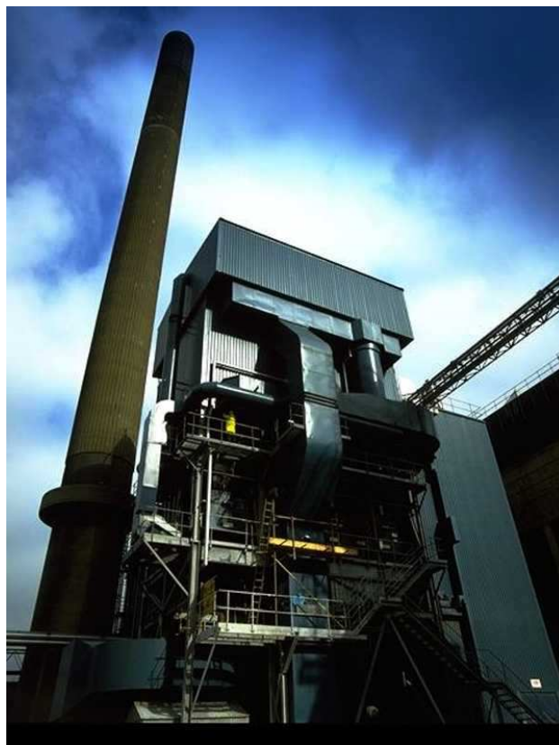
Fig 4 Nottingham Incinerator (c) Environment Agency
